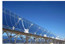
Concentrated Solar Power (CSP)
