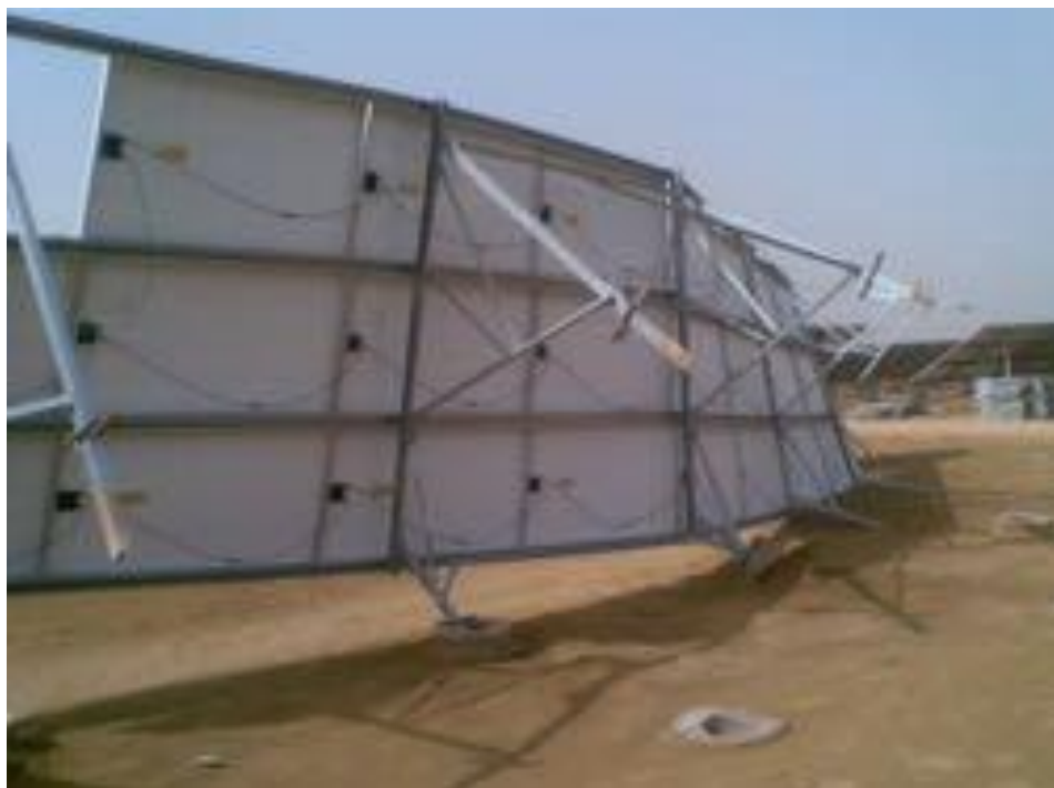
Poor quality structure and foundation
