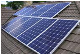
Solar Photovoltaic (PV) Systems
