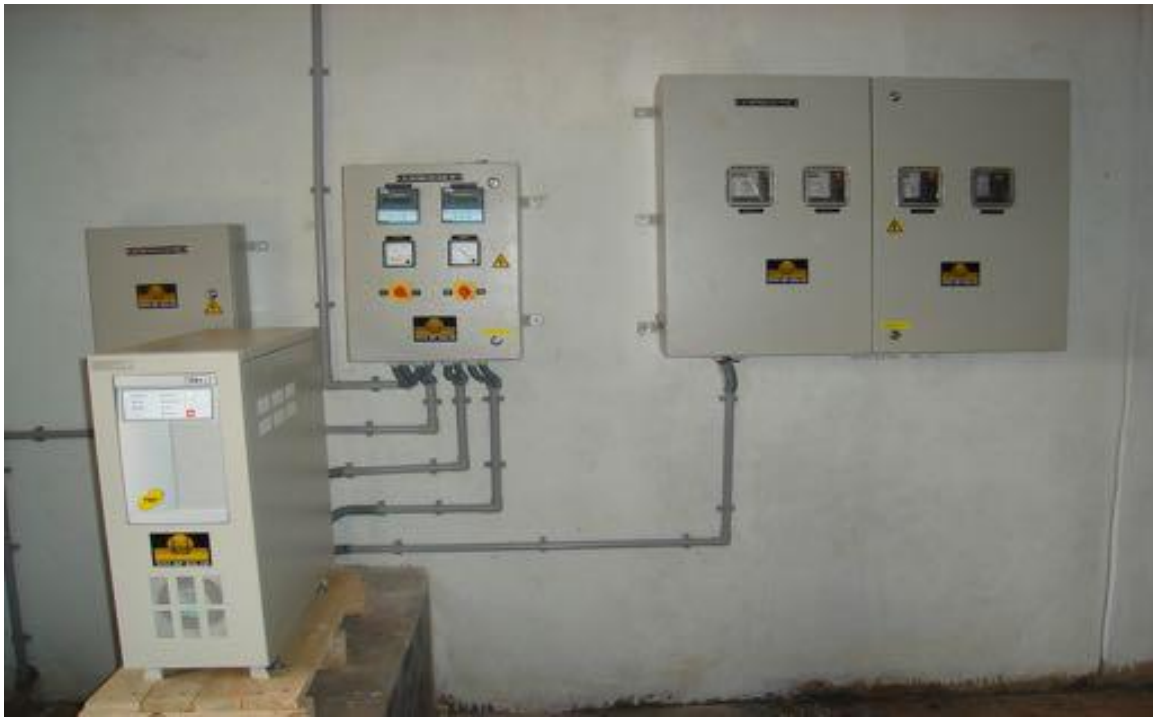
Example of control centre wiring
