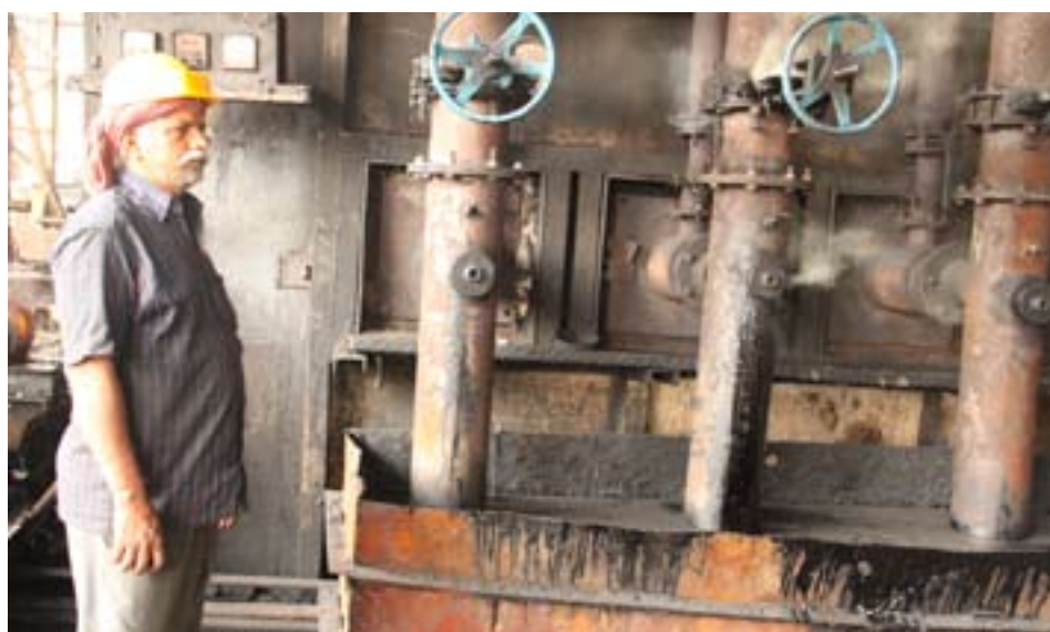
Front view of the energy-efficient re-heating furnace at Pulkit Steel Rolling Mills, Puducherry
