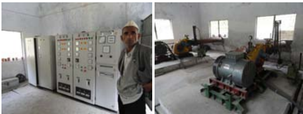
Control panel and turbines of the Jakhana micro hydel project
