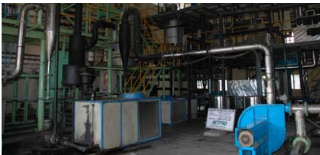
Biomass gasification system
