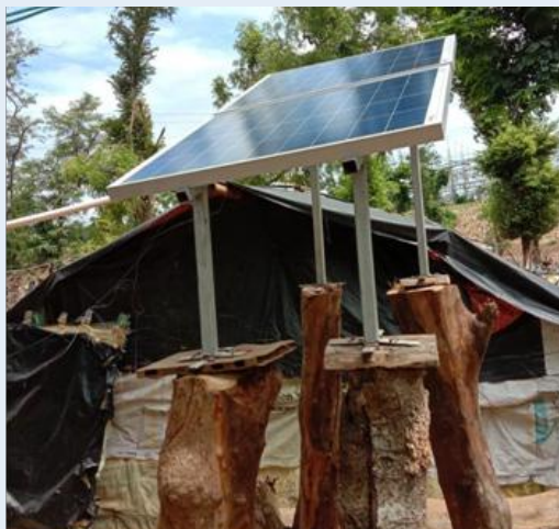
A micro grid for quick restoration of electricity
