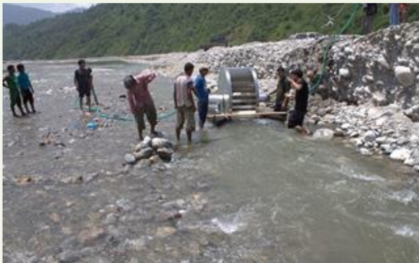
A Barsha Pump in operation
