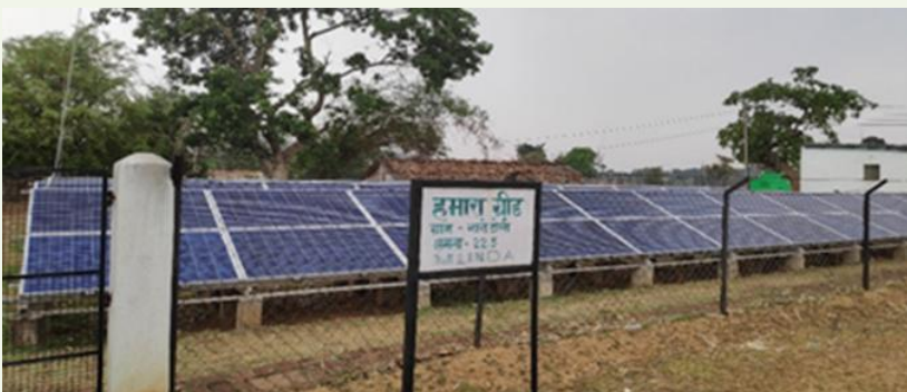
A community-based solar mini grid installed by Mlinda
