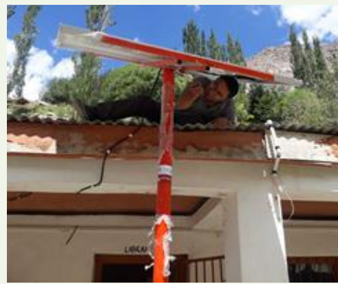
Solar Panels for Computer Labs
