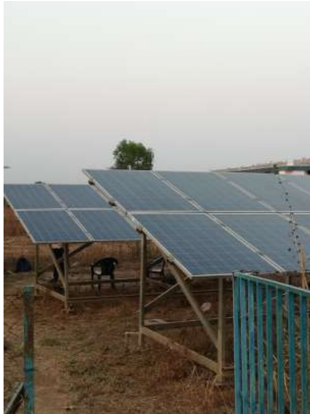
Figure 61 Solar panels at Site 1 (source: CES)
