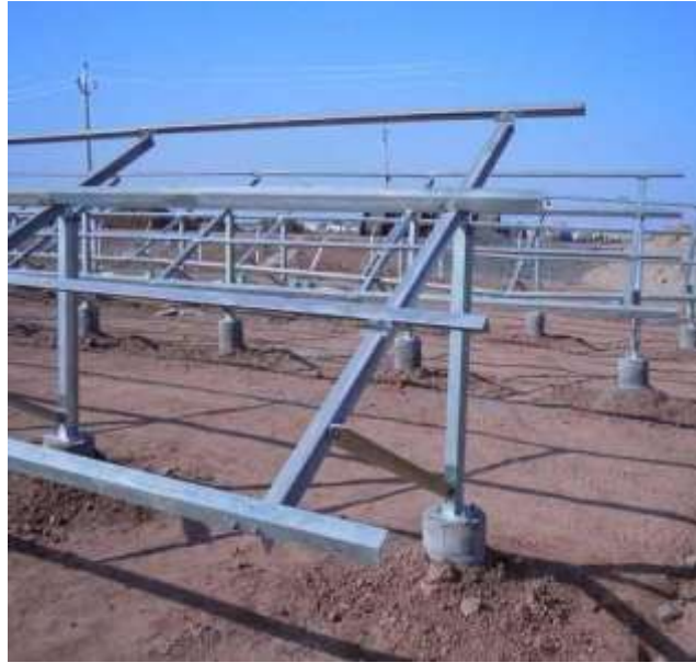
Figure 8 Solar PV Mounting Structure (source: IndiaMart)
